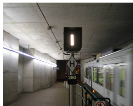
LRT Signalling Manchester
