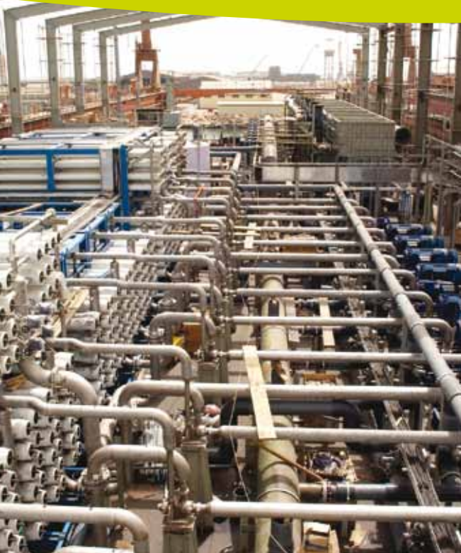
Shoaiba barge RO, Saudi Arabia. We were appointed owner's engineer by International Barges Company for Water Desalination (IBCWD).
