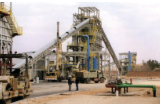
Our role in project managing the Egypt Float Glass Company's US$105 million plant near Cairo – in partnership with Arab Consulting Engineers – ranged from evaluating turnkey bids and reviewing designs to managing construction and co-ordinating a multi-disciplinary international team of contractors and suppliers
