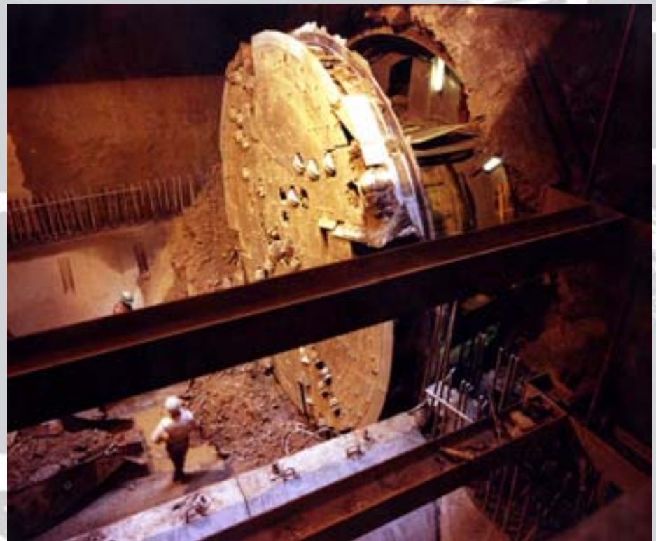
To relieve commuter congestion in central Melbourne we were part of a team which carried out a planning study followed by detailed design and construction supervision of four 3 km rail tunnels, 730 m of two-track viaduct and three stations for the city's underground rail loop
