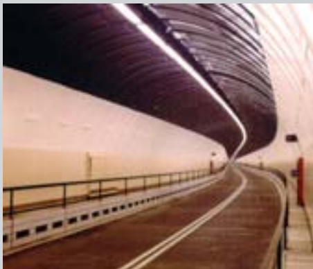
Following on from the Mersey Queensway tunnel, we were commissioned to plan and design the twin Kingsway road tunnels completed in 1974
