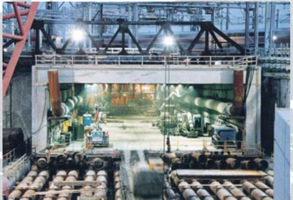
On the world's biggest tunnel jacking scheme – part of Boston's Central Artery project in the USA – three huge concrete tunnels carrying Interstate Highway 190 under eight live rail lines were built without any interference to rail services
