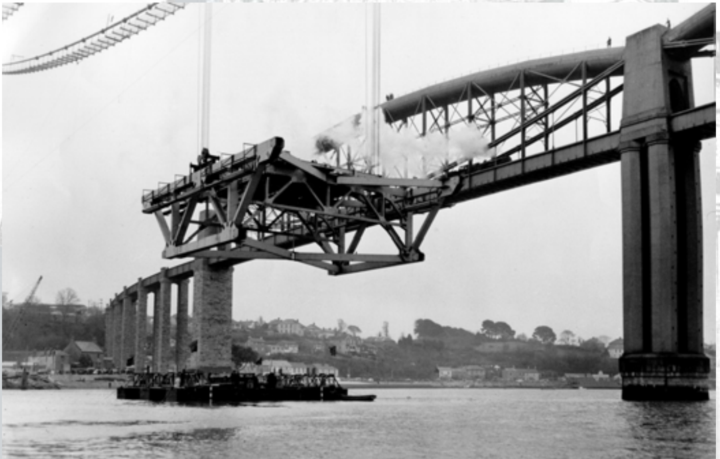
Located alongside Brunel's railway bridge, which opened in 1859, the Tamar suspension bridge, constructed 100 years later, has a main span of 1100 ft and carries a 33 ft carriageway with two 6 ft footpaths over the River Tamar. Sections weighing some 80 tons were floated out on the river and raised into position using winches connected to the main cables
