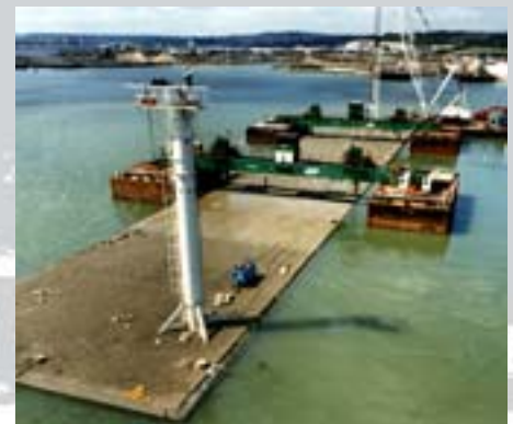
Our cost-effective and innovative design for the Medway Tunnel in Kent, UK, comprised cut-and-cover approaches and a 370 m long twin-bore immersed tube tunnel designed to be watertight without an external membrane
