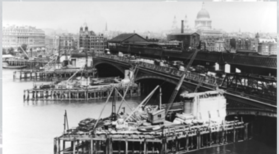
The firm's work on the widening of Blackfriars Bridge in 1908 was the start of a long association with the Corporation of London
