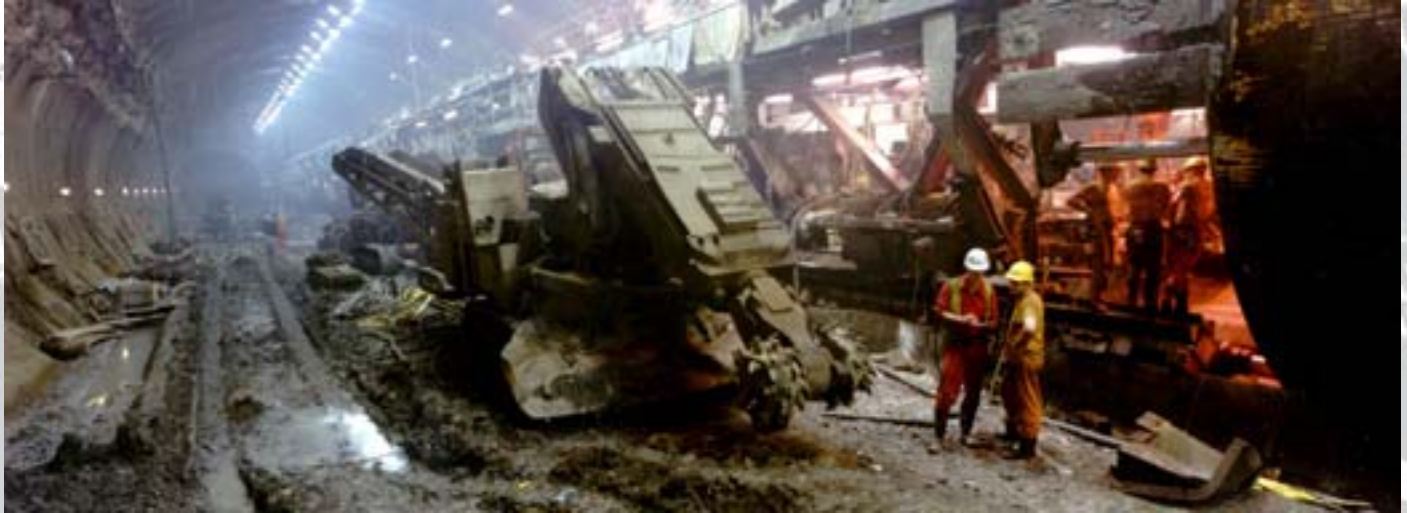
We were principal design consultant for all civil and geotechnical engineering on the UK section of the Channel Tunnel. This included the award-winning 156 m long, 18 m wide and 10 m high cross-over cavern – the world's largest subsea excavation – constructed using the New Austrian Tunnelling Method
