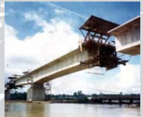
Malaysia's Kuala Lepar Bridge across the Pahang River was one of several bridges we designed in the 1970s using the balanced cantilever method of construction
