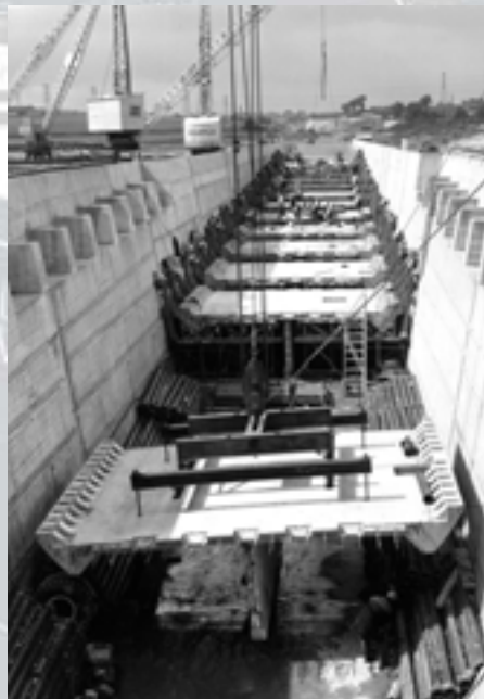
The 4688 ft long Dartford Tunnel under the River Thames near London had a road deck formed by pre-cast reinforced concrete units weighing 37 tonnes each
