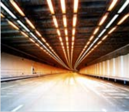
We worked on various phases of the M25, London's orbital motorway, designing viaducts, bridges and sections of highway as well as in-tunnel services such as lighting, ventilation and emergency communication systems
